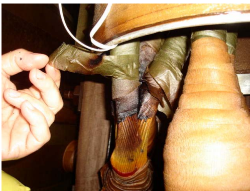
Fig. 7. Burning of solid insulation (paper)
