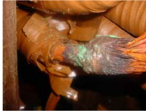
Fig. 8. Heating indications in the interconnection cable of tap changer
