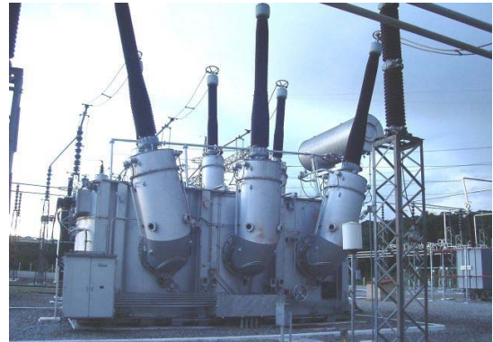
Fig. 6. Three-Phase Autotransformer used in Case Study 2
